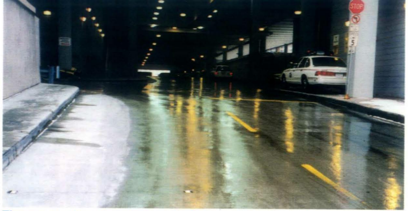
The snowmelt system was applied on ramps to the underground parking garage and on pedestrian and handicapped access ramps.
