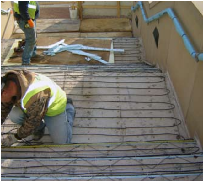
The M.I. snow melting cable assemblies are tied to rebar before the concrete is poured.
