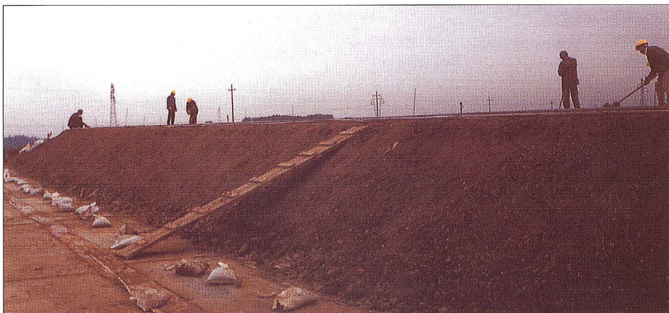
Italian construction workers prepare the soil for Delta-Therm's mineral insulated heating cable on BioPile No. 1. The photo shows the third of six total levels.
