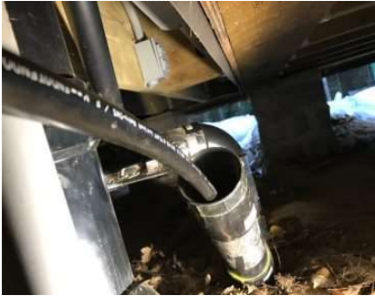
Illustration #10: SR Cable Inside of Metal Conduit Buried in Subsoil
