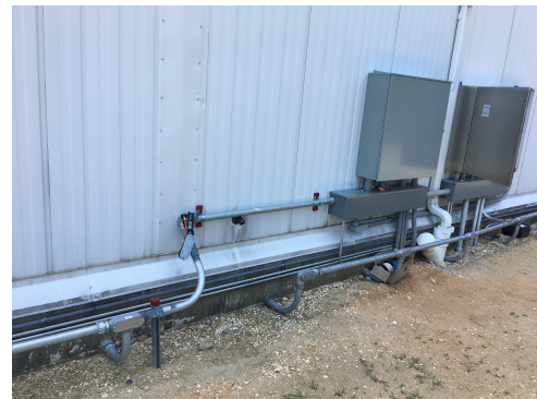
Illustration #6: Frost Heave Prevention Installation: Freezer floor subsoil conduit runs stubbed outside. 90 degree elbows attached to facility conduit system.
