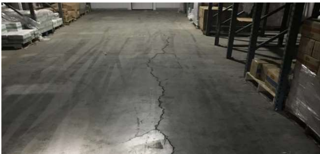
Illustration #4: Frost Heave in Cold Storage Facility Floor
